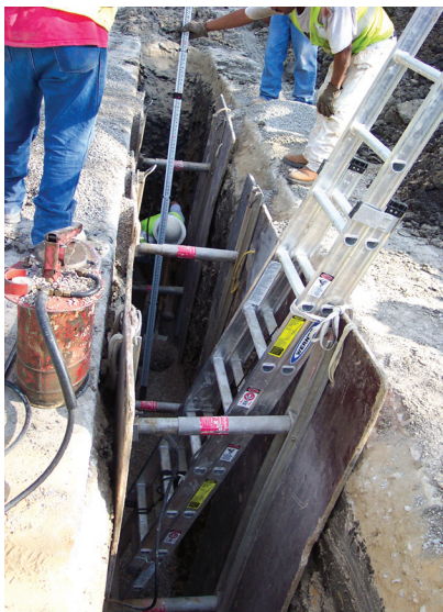
Figure 1. Work crew installing water pipes. Aluminum hydraulic shoring is being used as a protective system for the trench. Photo courtesy of George Kennedy, NUCA.
